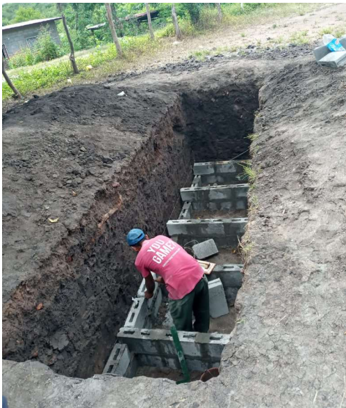
Digging out and building the pits for double-pit latrines in San Agustin.
