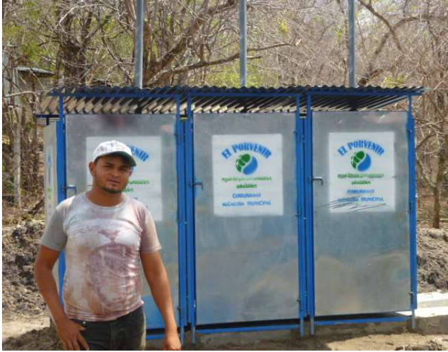
One of the parent volunteers who helped construct the double-pit latrines in Puertas Viejas.
